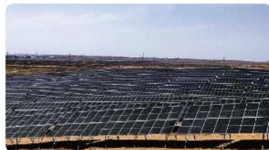
250MW Ningdong Hybrid PV Plant Ningxia · China Utility
