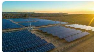
1.5MW Setta PV Plant Pernambuco, Brazil Utility
