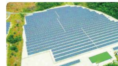
3.24MW Kanzaki PV Plant Kanzaki · Japan Utility
