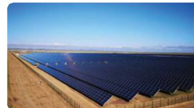
50MW Suntech's First Kazakhstan Project Karaganda · Kazakhstan Utility
