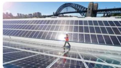
384KW | Sydney Theatre Co Rooftop PV Project Sydney · Australia | Commercial and Industrial Rooftop
