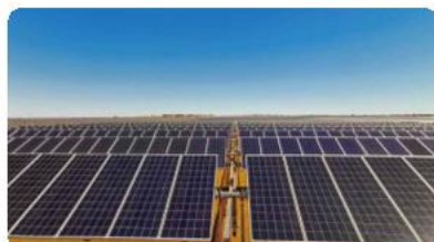
250MW Kimberly Droogfontein PV Plant South Africa Utility
